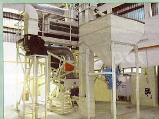
Overall view of the new installation.
