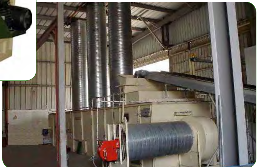
Conveyor Drier with stainless steel contact parts, fed by Belt Conveyor
