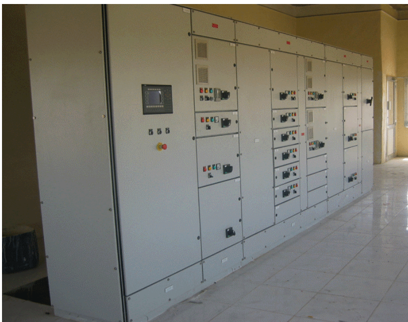
PLC Control Panel with SCADA system (Sudan)
