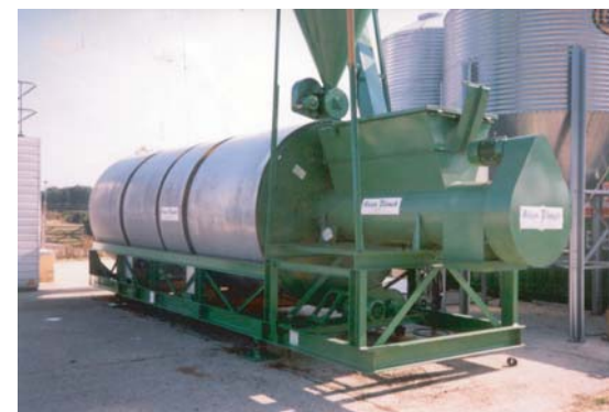
Rotary waste drier used to dry sludge
