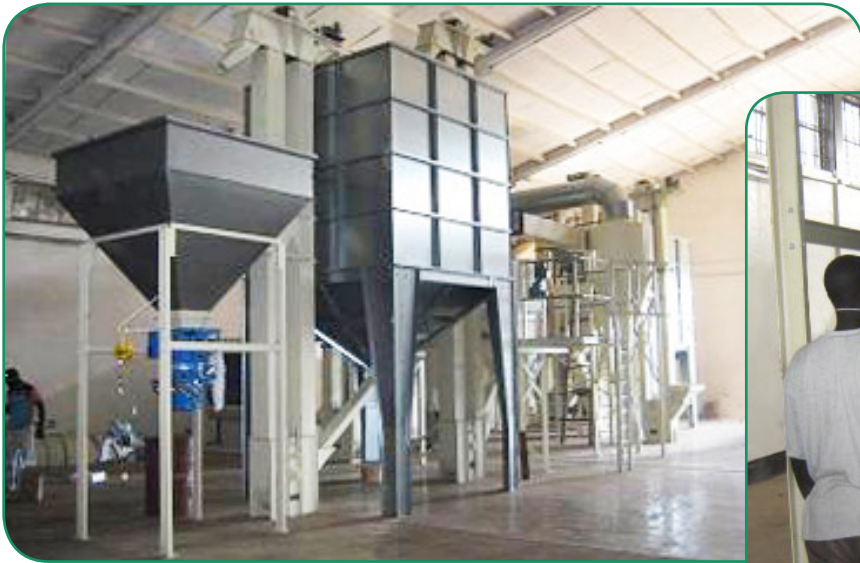
Sacking hopper with pre-sacking bin
